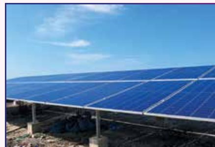
180kWp Grid Connected Roof Top Solar Power Plant at District Hospital Aluva Site : District Hospital Aluva Cost : ₹63 Lakhs
