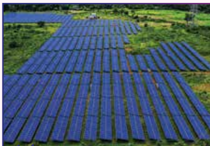
3500kWp Grid Connected Ground Mounted Solar Power Plant Site : 220kV substation KSEBL Mylatty, Kasaragod Cost : ₹17.5 Cr
