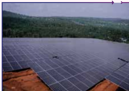
20.5MWp Ground-Mounted Solar Power Plant at INKEL Greens, Malappuram Kerala's First Group Captive Project
